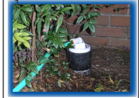
Step 5. Align the garden hose and extension cord neatly across the parking lot, as shown in the photo. Locate the sewer cleanout in the planter bed below the wall with the drive-thru window. Attach the white cleanout cap to the cleanout. Attach the garden hose to the cap as shown.
